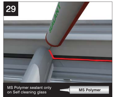
Seal along the ridge baffle where it meets the glazing and over any bar where it meets the ridge.
